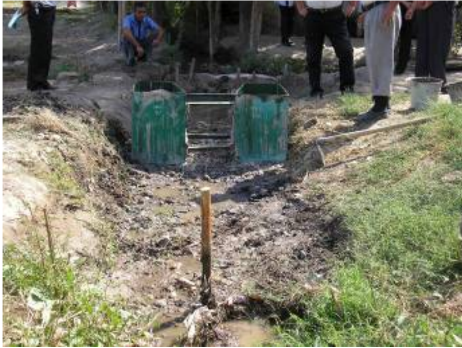
Figure 1.9. Putting metal form for a SANIIRI flume along the canal section centerline.
