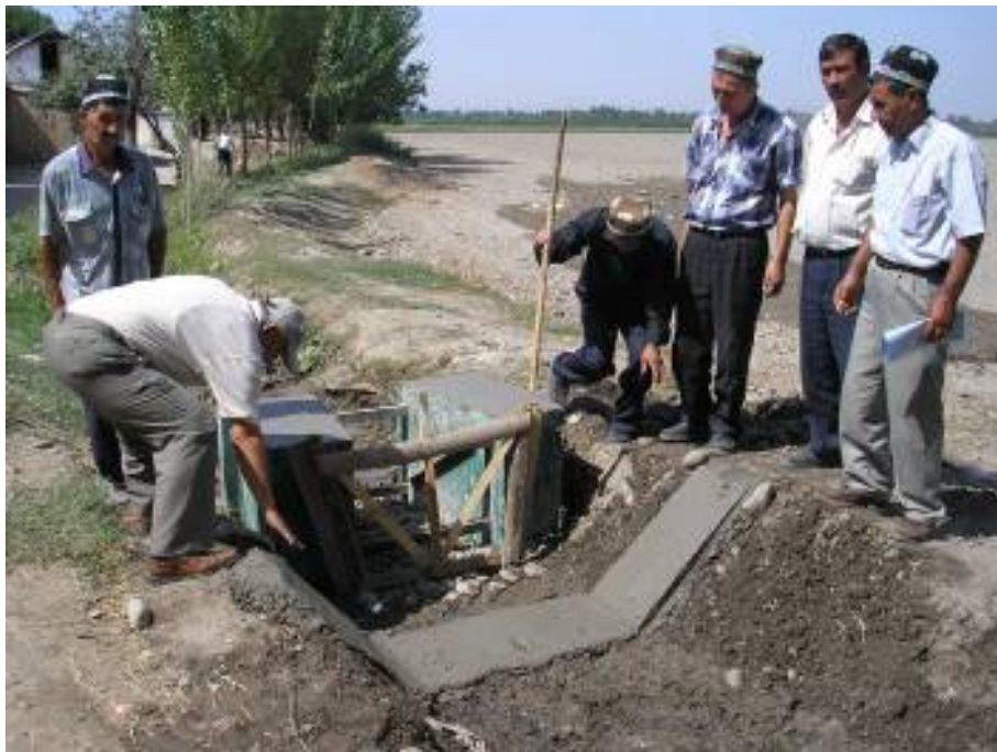
Figure 1.10 Part of the concrete lining of the intake channel of a gauging station with a SANIIRI flume.
